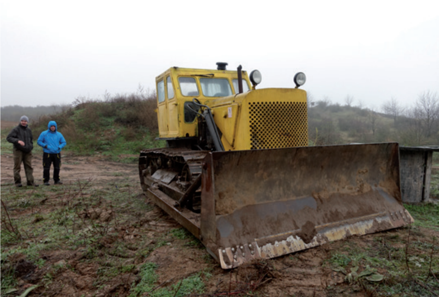
Fig. 7: Turf removal in order to remove expansive wood small-reed on the most affected areas. (Photo: Beleco, 2018)
