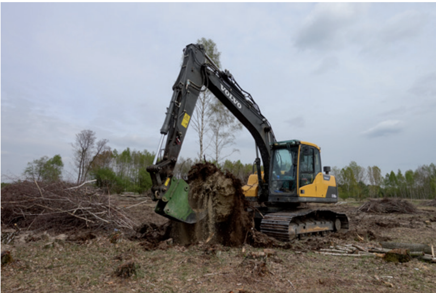
Fig. 4: Removing stumps on Pánov using a tracked excavator and special accessories. (Photo: Beleco, 2017)
