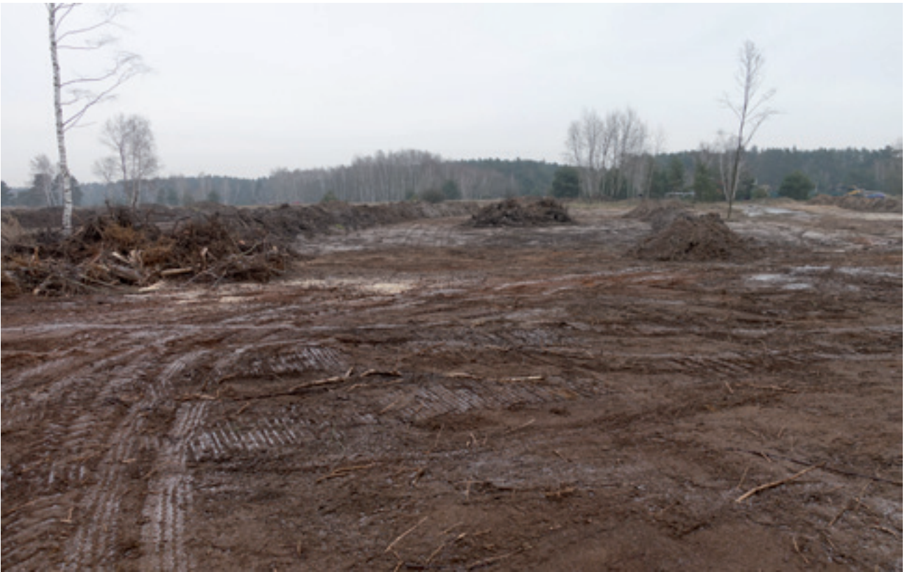
Fig. 9: After the initial remediation measures, some parts of Pánov looked like a lunar landscape. However, their thorough implementation was necessary for the success of the subsequent restoration management. (Photo: Beleco, 2017)
