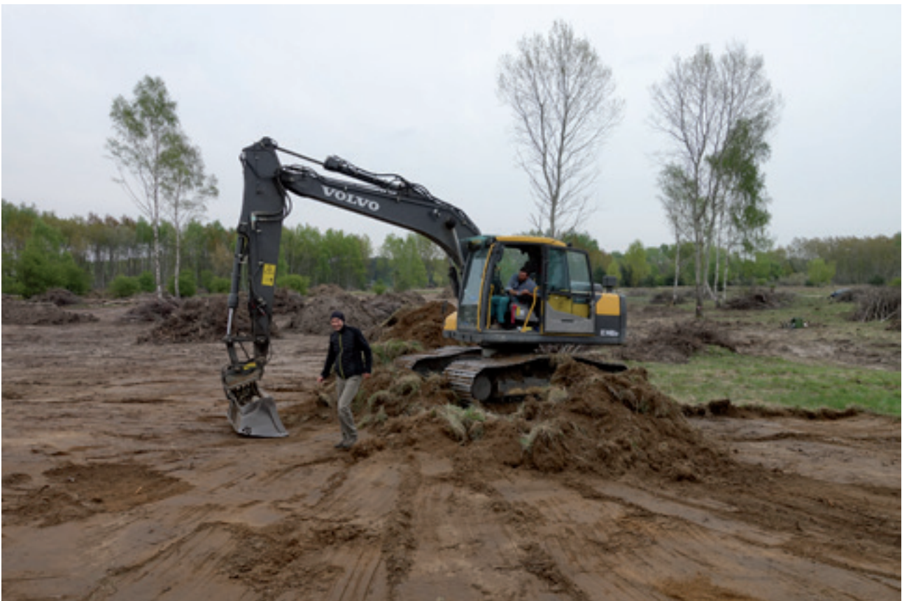
Fig. 5: Removal of the top layer of soil degraded by the rotten litter from self-seeding woody plants. (Photo: Beleco, 2017)
